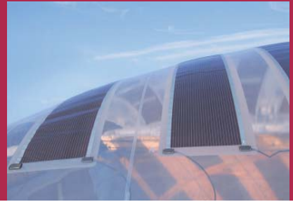
Atrium roofing with PV Flexibles on ETFE-membrane cushion
